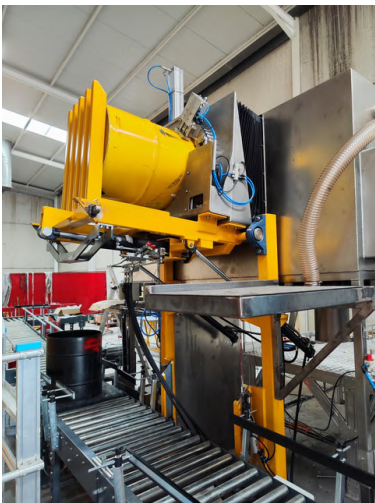
Radioactive waste sorting plant for South African Nuclear Energy Corporation
